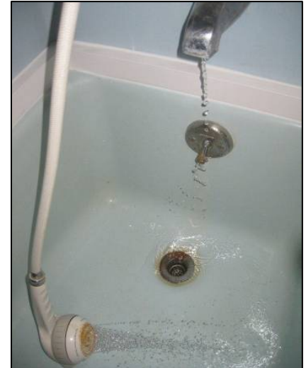
Figure 3: A leaking diverter allows water to flow out both the showerhead and the tub spout simultaneously.
