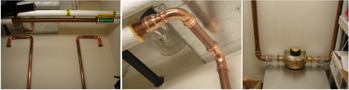
The above photographs show existing supply piping, piping modifications, and the new water meter.
